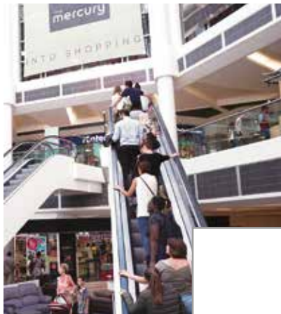
Lifts and escalators
